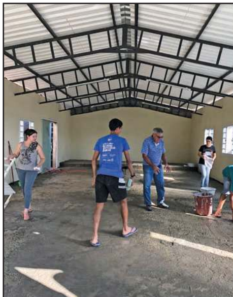
A construction team built a church in Pouso Alegre, Brazil, as part of the annual evangelism outreach in the country July 6-17.
